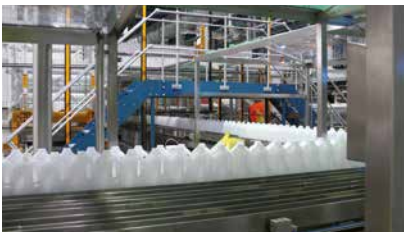
Intermediate Bottle Storage System – IBSS for buffering of empty plastic milk bottles. Balancing the difference between blow molder and filler to increase the capacity of the filler.
